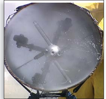
BJV cleaning pipe with four extensions added.
