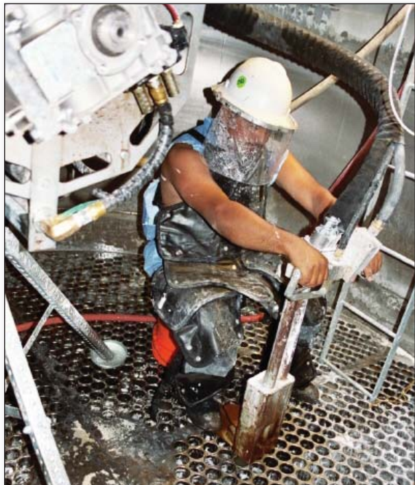
Reel eliminates hose hazard.
